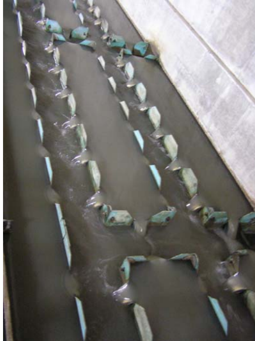
Figure 6. Primary clarifier effluent weirs with two clarifiers in service. (Clarifier 4 shown, SOR=1377-1442 gpd/ft 2 )
